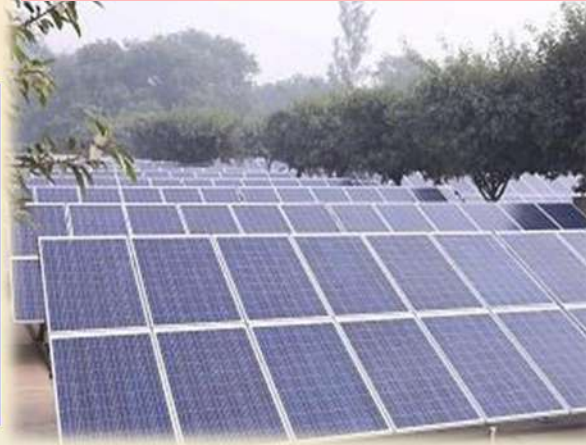
2 MWp Solar Power Plant at Burla
